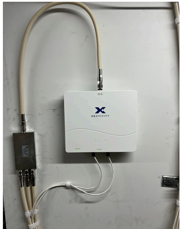
Above: Coverage unit located in the second floor IT closet.
