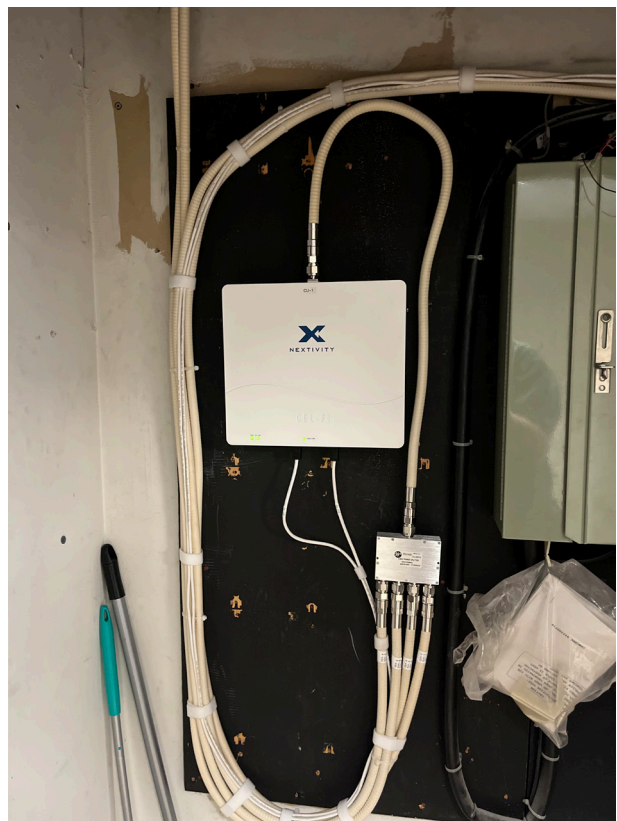
Above: Coverage unit located in the first floor IT closet.
